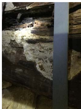
Figure 2: an important fungal rot at a tie-beam rafter joint. The external appearance does not allow to infer the real residual cross section.
