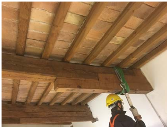
Figure 1: operators must have a safe access to the structures
